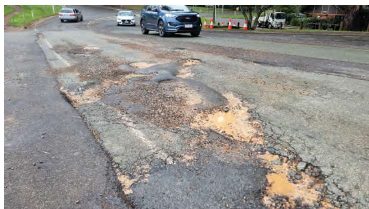
Main Street's finest... the busiest intersection on the Mountain, and still the direct route for dozens of fully-laden water tanker movements each week.
