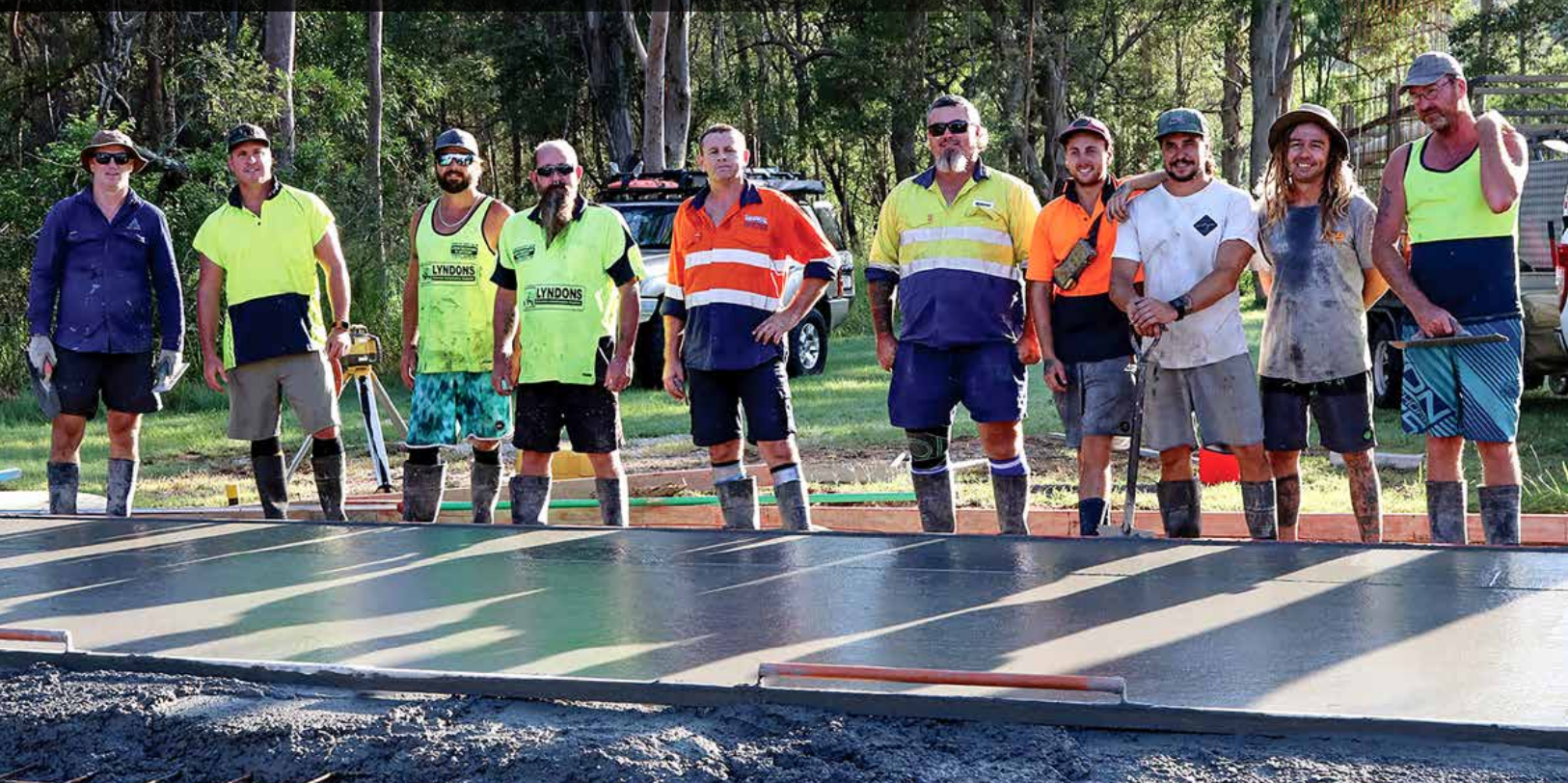
Tamborine Village Lions Club members put in a mighty effort to lay the foundation for their new security storage shed which was completed just before the COVID-19 lockdown was put in place. More photos Page 4.
